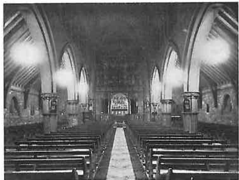
ST. ANDREW'S CHURCH, PLAISTOW. New lighting by means of eight 4-light Corona fittings, equipped with 60-watt Mazda lamps and Opalux reflectors. Note the improved appearance of the interior and the way the Altar stands out.
